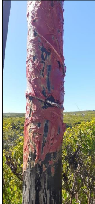
Figure 9. Greasing of problematic electrical poles remains ongoing until a long-term solution can be implemented.
